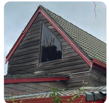
✔ Cracks or Cupping Wood
